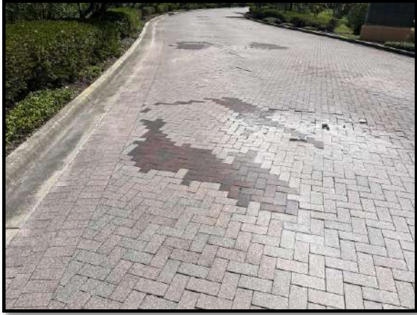
Figure 9 – Damaged pavers at Cory Lake Boulevard
