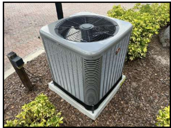
Figure 2 – New condensing unit at gatehouse
