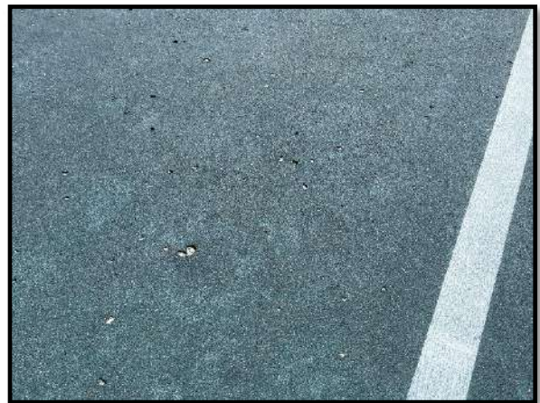
Figure 8 – Holes in tennis court surface
