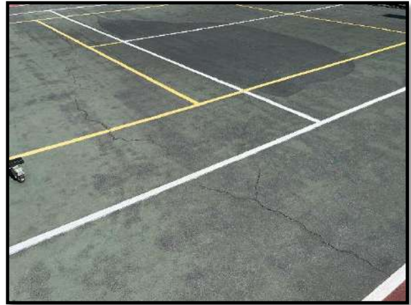
Figure 6 – Large pickleball/tennis court cracks
