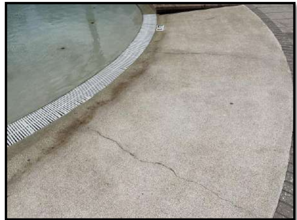
Figure 2 – Plaster finish cracks
