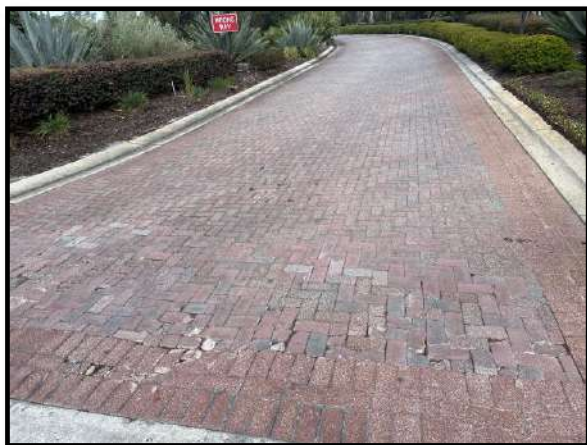
Figure 1 – Damaged pavers at southeast entrance
