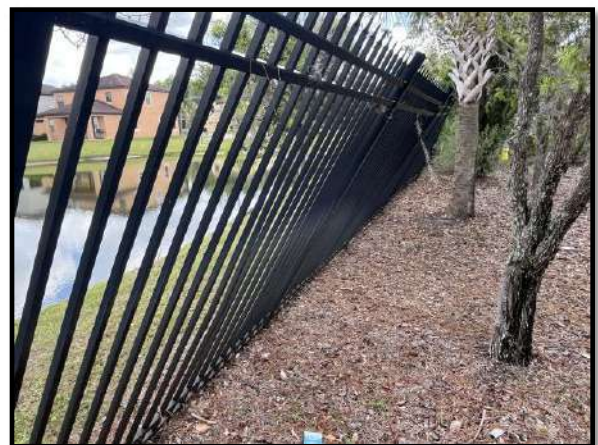
Figure 2 – Leaning section of aluminum fence
