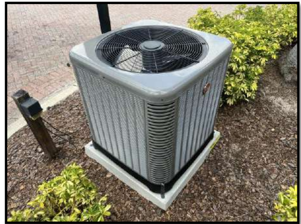
Figure 2 – New condensing unit at gatehouse
