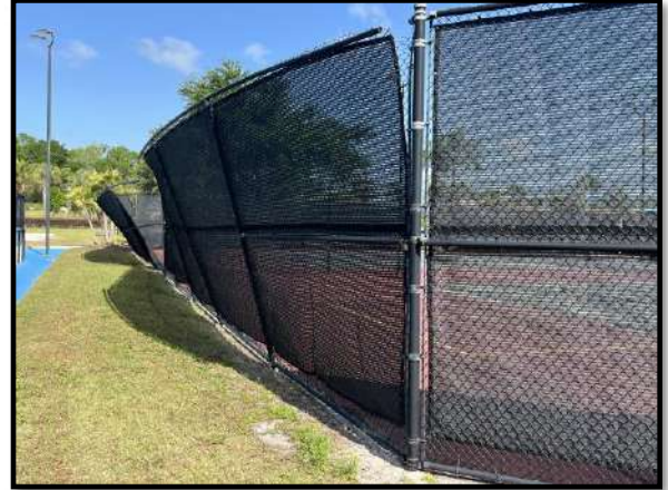
Figure 2 – Falling fence at pickleball/tennis courts
