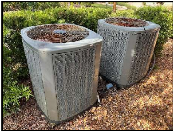
Figure 1 – Condensing units at the Beach House
