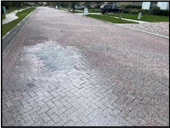
Figure 11 – Paver settlement at Cory Lake Drive
