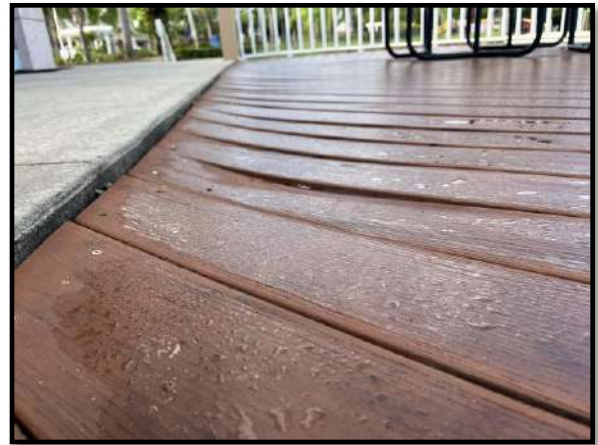
Figure 2 – Warped deck board
