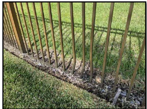
Figure 2 – Isolated fence damage by water slide
