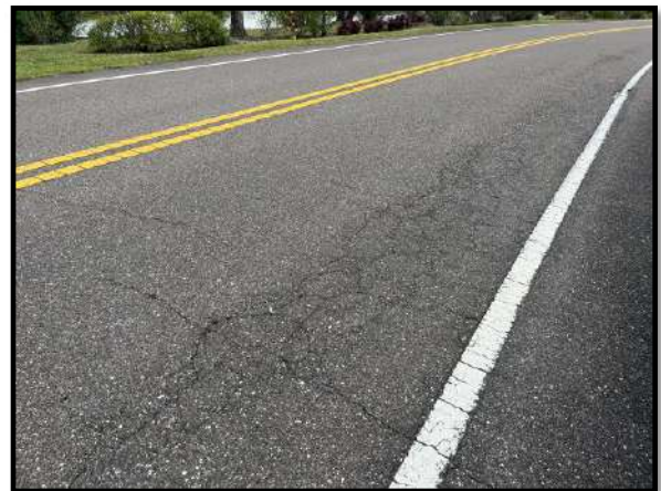
Figure 2 – Alligator cracking at Cory Lake Drive
