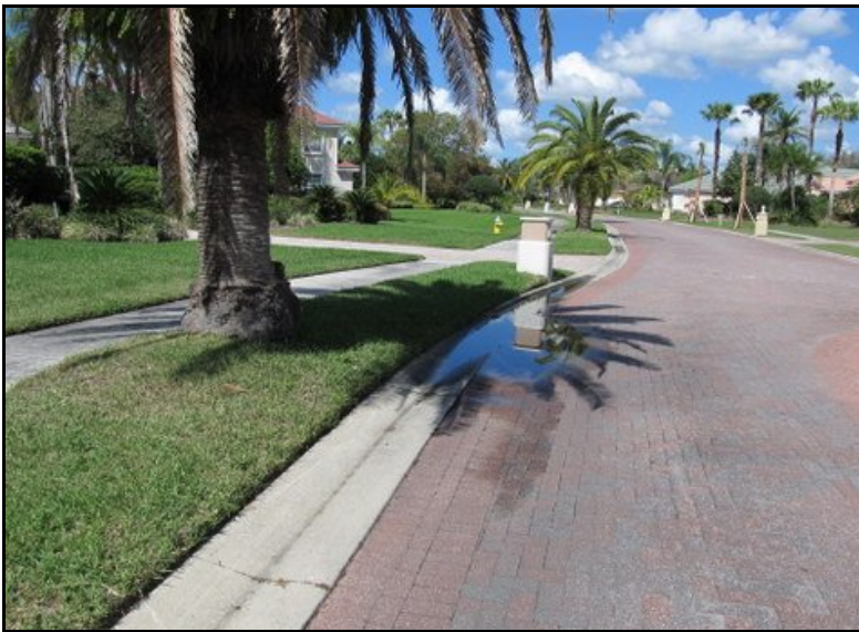
Concrete curb and gutter - Note drainage issue
