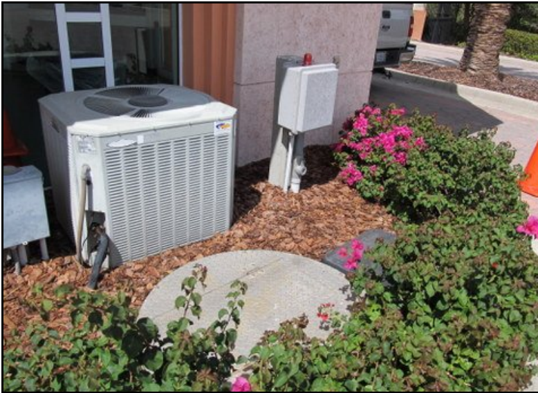
Building services at gate house
