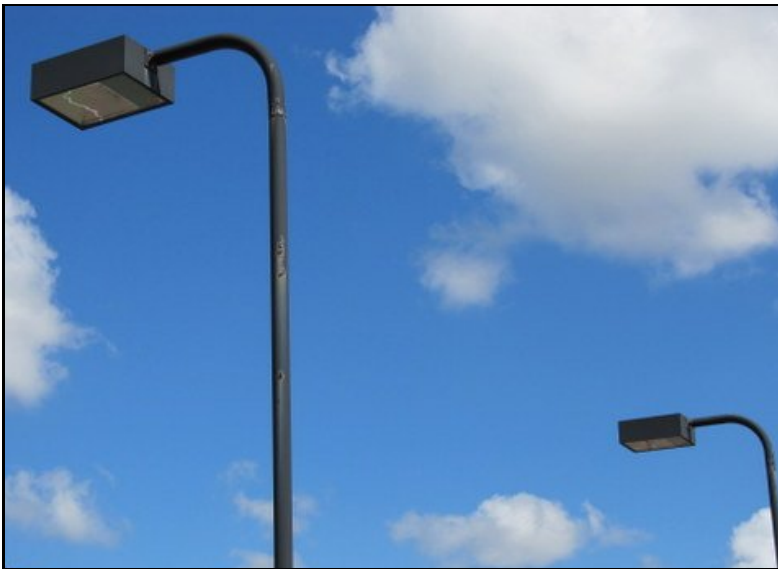
Light poles and fixtures at courts
