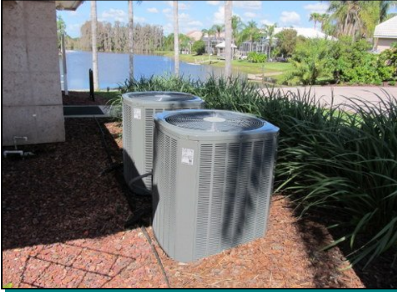
Beach house building services
