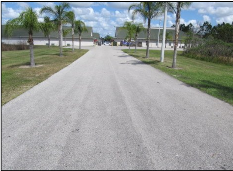
Asphalt pavement adjacent to Cory Lake Drive Maintain through the Operating Budget
